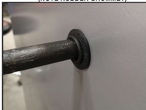
FIGURE 28 - FURNACE GAS PIPE CONNECTIONS (NOTE RUBBER GROMMET)
